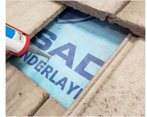
4. Remove hook, clean debris, then fill pilot holes and rib on back of hook with roofing sealant.
